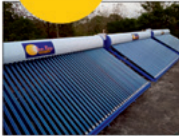
Solar Water Heater
